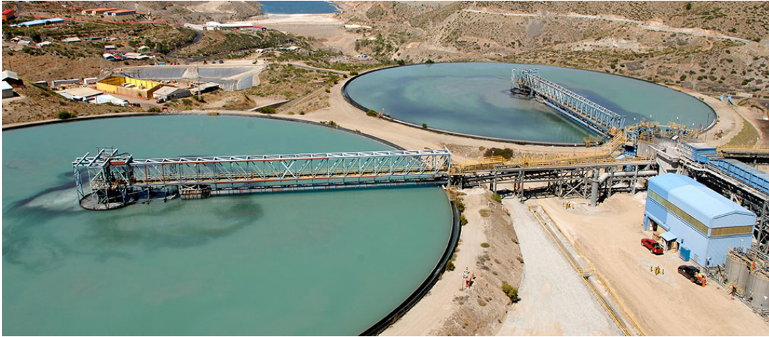
Figure 3: Salamanca thickeners. Both units presents a short-circuit in gray color at center Reprinted from CENTRA Ingeniería Adquisiciones Construcción, by CENTRA Ingeniería Adquisiciones Construcción, Retrieved October 20, 2018, from http://www.centra.cl/construction-en/mining3-en/ . Reprinted with permission.
